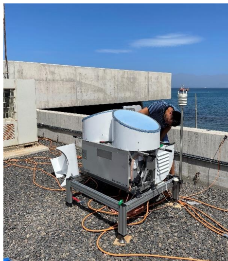
Figure 30: The installation of the 94 GHz FMCW Doppler Cloud Radar on the rooftop of the OSCM, Cape Verde.
